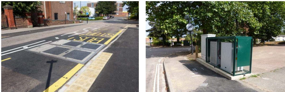
Figure 14: Example of IPT Technology WPT chargers installed in Milton Keynes
