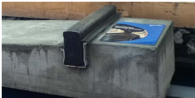
Figure 24: Balfour Beatty embedded rail system
